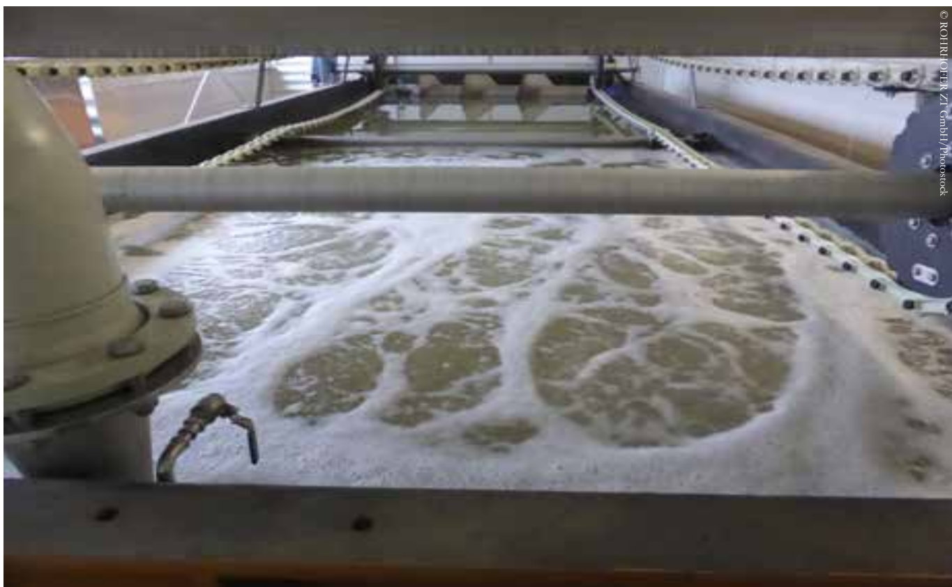
Pre-aeration and sedimentation tanks
