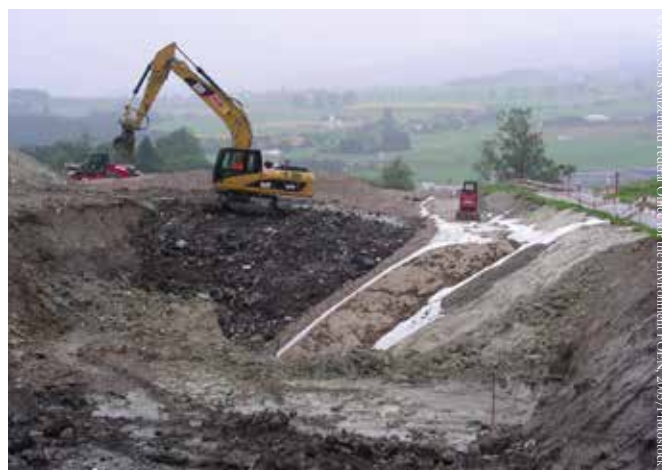
Construction of a lateral mineral seal system to prevent slope water from entering the landfill
