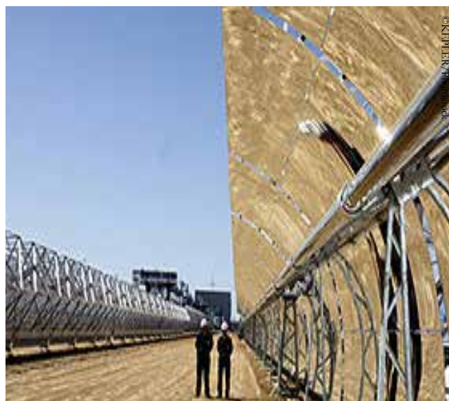
View of the Solar Plant
