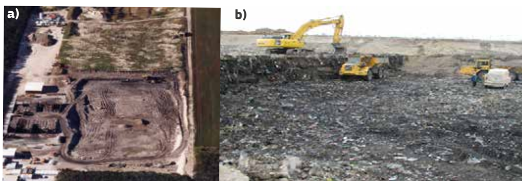
From left to right: a) Aerial view of the site at the beginning of the clear-up operations b) Excavation of municipal waste with a skeleton-excavator
