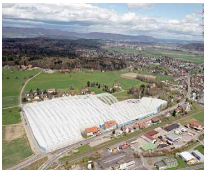
The site of the Kölliken hazardous waste landfill showing complete enclosure for the remediation works (2007- 2018)
