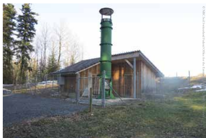
Gas flare facilities.
